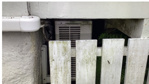
Varmepumpe under terrasse
