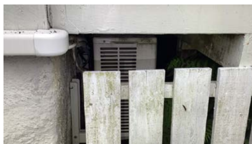
Varmepumpe under terrasse
