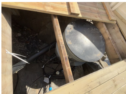
Pumpe kum, plassert under terrasse.
