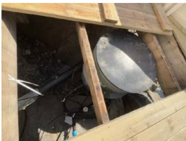
Pumpe kum, plassert under terrasse.
