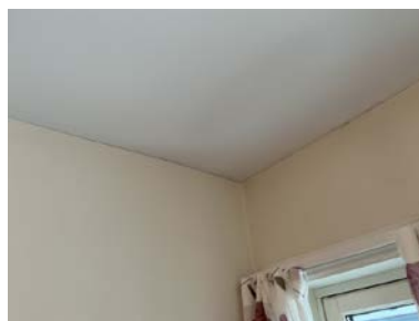
Riss i overgang vegg/himling.
