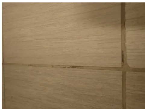
Riss i flisfuger.
