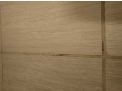
Riss i flisfuger.
