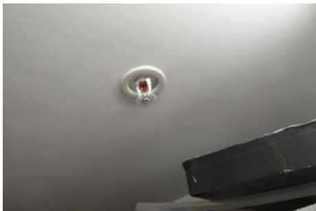
Sprinkelhode i himling.
