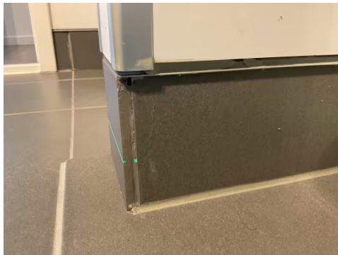
Sprekker i fug.
