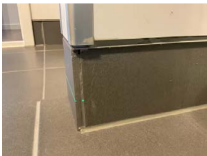
Sprekker i fug.
