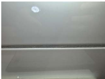
Riss i veggflis over servant.
