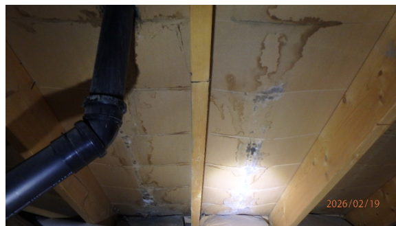
Fuktflekker i undertak
