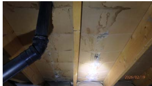
Fuktflekker i undertak
