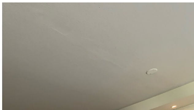
Ujevnheter i himling.
