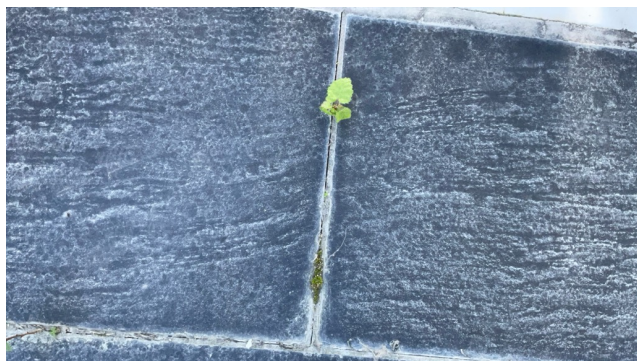
Sprekker i flisfuger.
