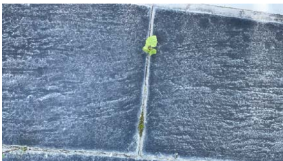
Sprekker i flisfuger.
