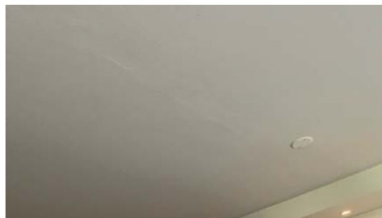
Ujevnheter i himling.
