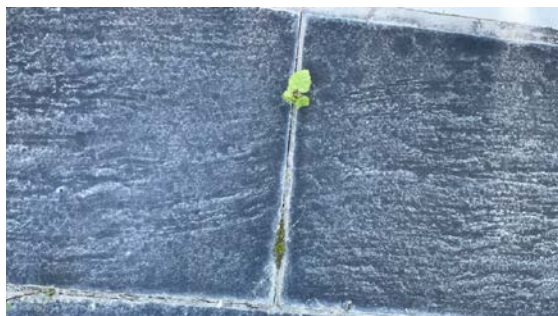
Sprekker i flisfuger.
