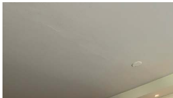
Ujevnheter i himling.
