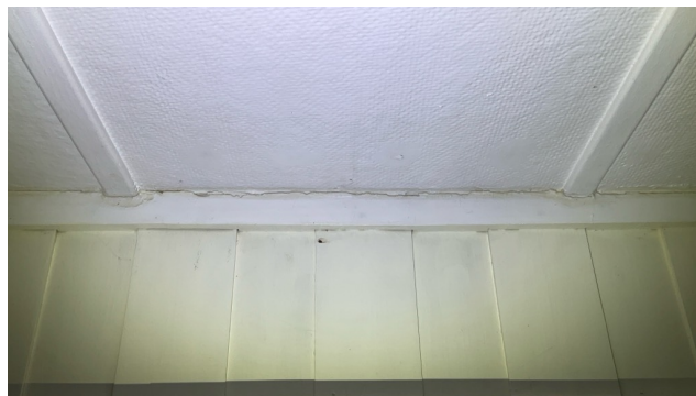
Riss overgang vegg/himling
