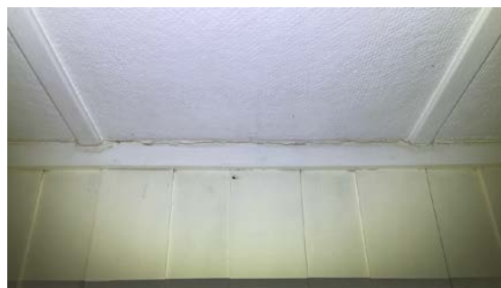
Riss overgang vegg/himling
