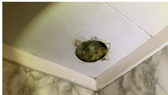
Ventil mangler i himling.
