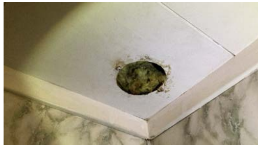
Ventil mangler i himling.
