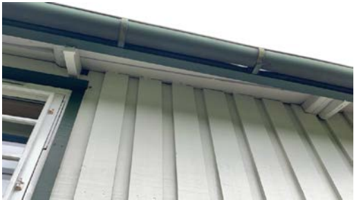
Begrenset ventilering langs raftekasse
