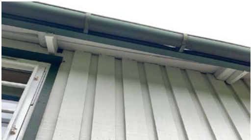
Begrenset ventilering langs raftekasse
