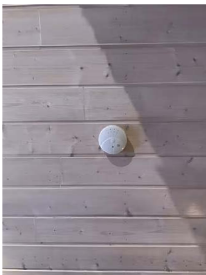
Viser brannmelder i himling.
