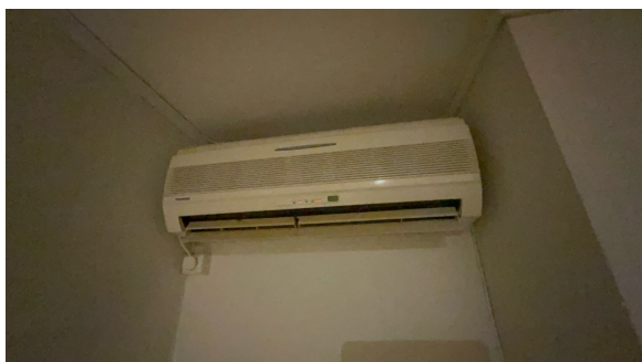
Varmepumpe, innvendig aggregat.
