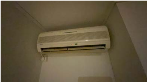
Varmepumpe, innvendig aggregat.
