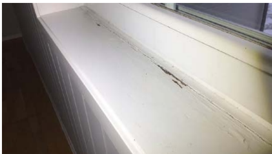
Fukt merker i foring i underkant
