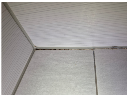
Sprekker i mykfuge.
