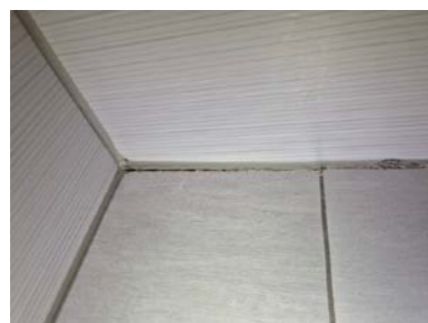
Sprekker i mykfuge.
