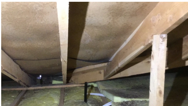
Fuktskader i undertaket
