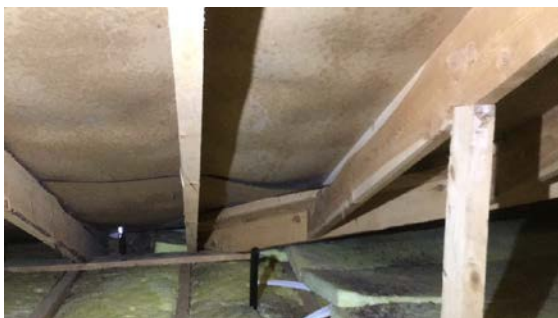
Fuktskader i undertaket
