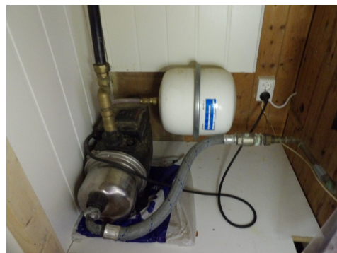
Vannpumpe i bod.
