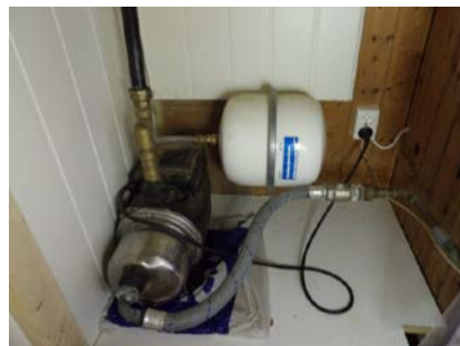
Vannpumpe i bod.
