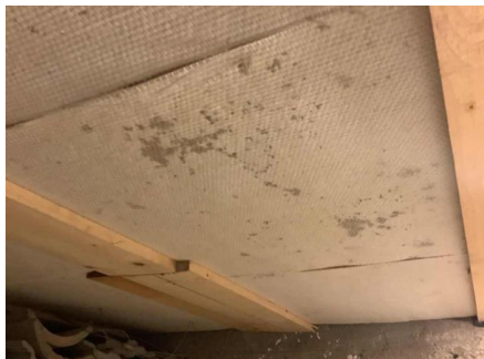
Misfarging i himling.
