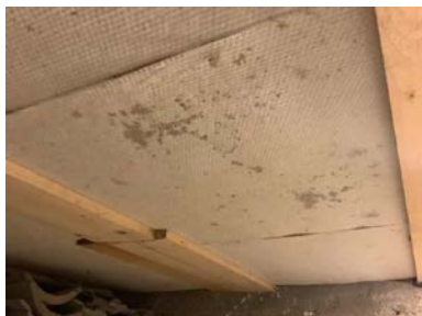
Misfarging i himling.
