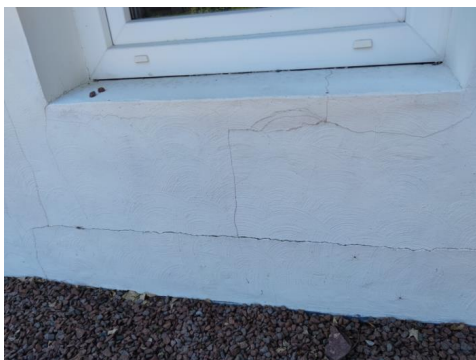
Sprekker i puss.
