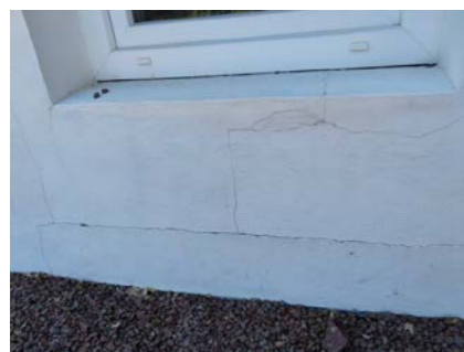
Sprekker i puss.
