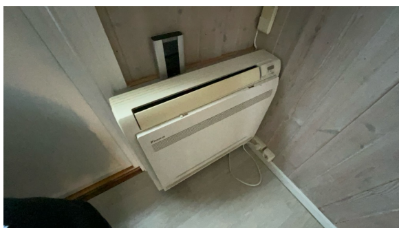
Varmepumpe, innvendig aggregat.
