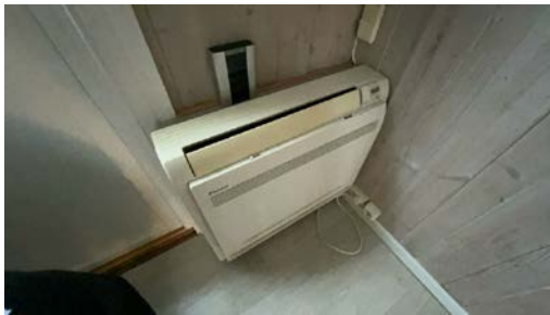
Varmepumpe, innvendig aggregat.
