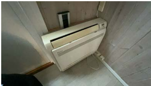
Varmepumpe, innvendig aggregat.
