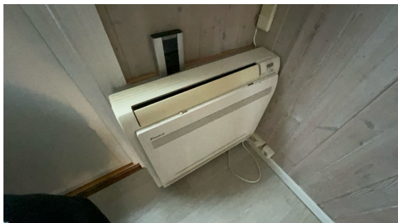
Varmepumpe, innvendig aggregat.
