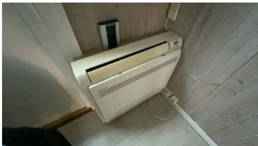
Varmepumpe, innvendig aggregat.
