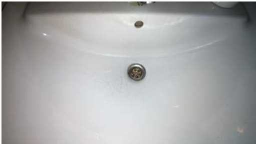
Riss i servant
