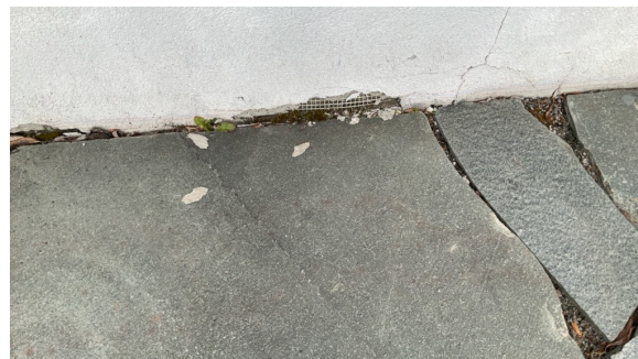
Noe manglende puss.
