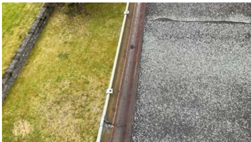
Noe rust i takrenner.
