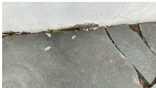
Noe manglende puss.
