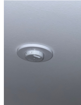
Innfelt sprinkelhode for slukking
