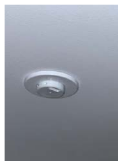
Innfelt sprinkelhode for slukking
