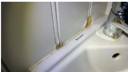
Fuktsvelling i veggplater over vask.
