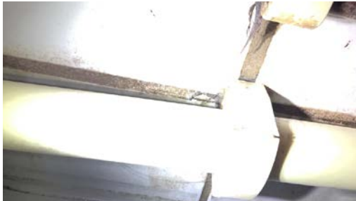
Riss i flisfuge.
