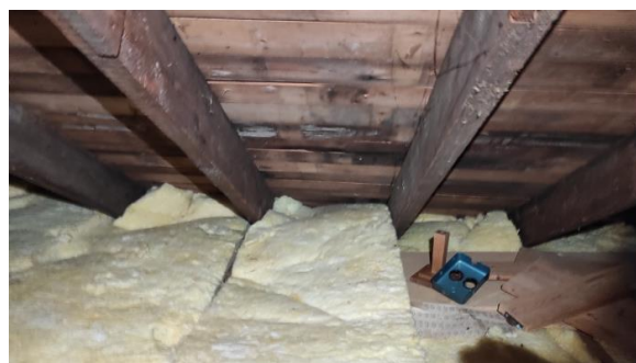
Manglende lufting i raft.
