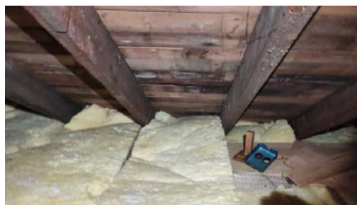
Manglende lufting i raft.
